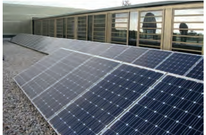
Solar panels provide some of the electricity used at The Bridge
