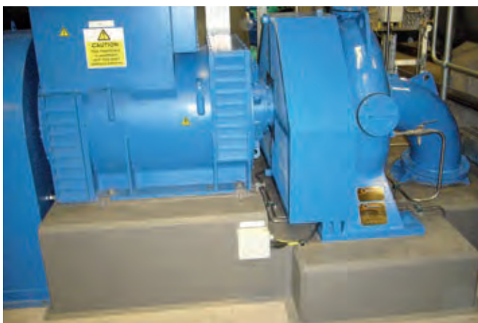
The new hydropower installation at Megget Reservoir
