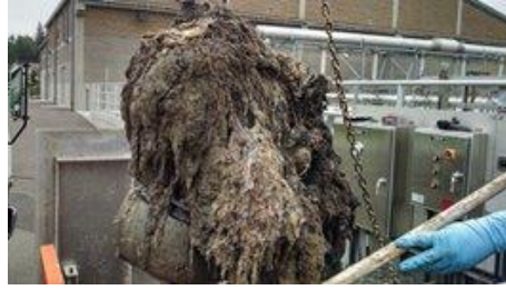
A pump in a sewer choked by wet wipes
