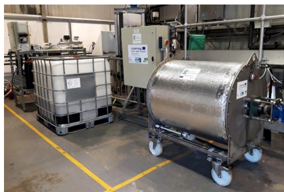
The microalgae reactor at the Bo'ness Testing Centre
